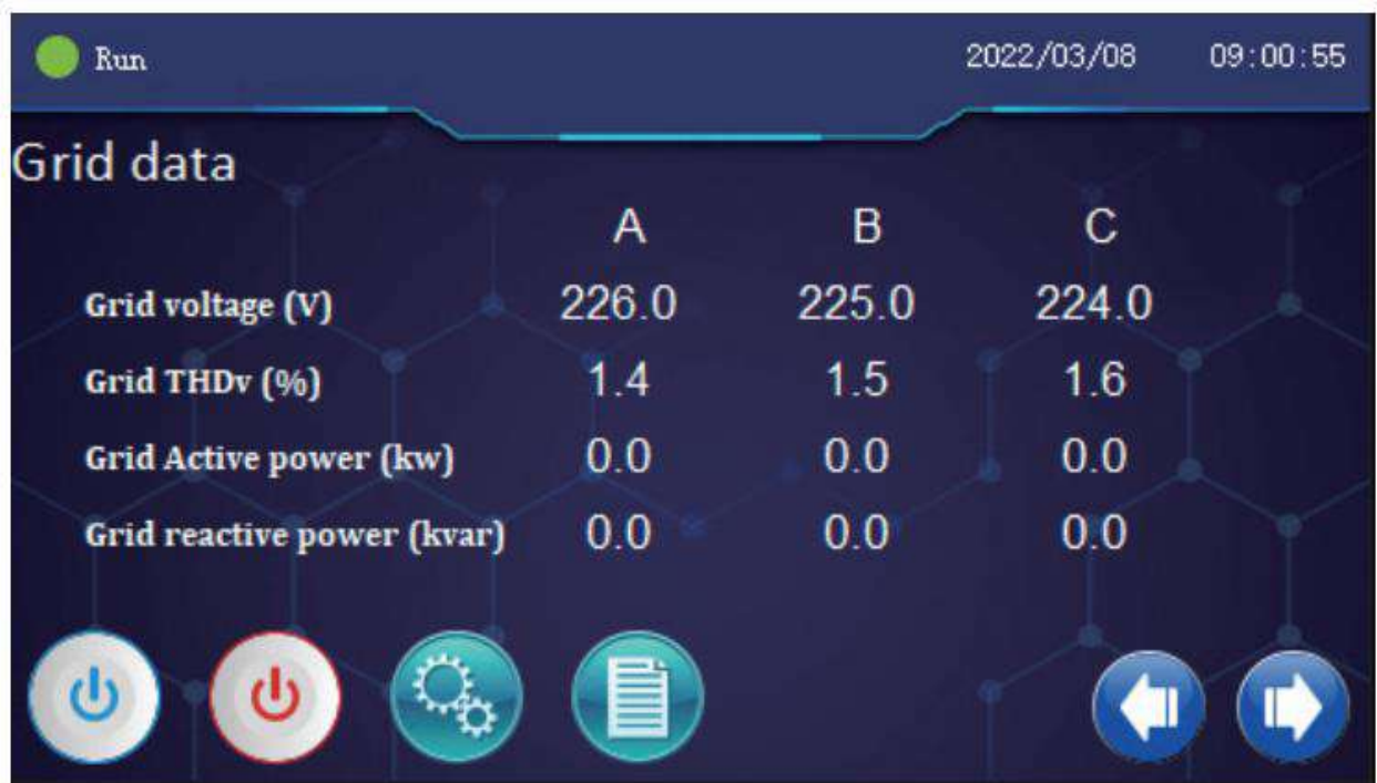
Figure 2 Touch screen main interface
